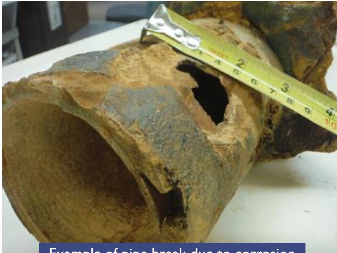
Example of pipe break due to corrosion
